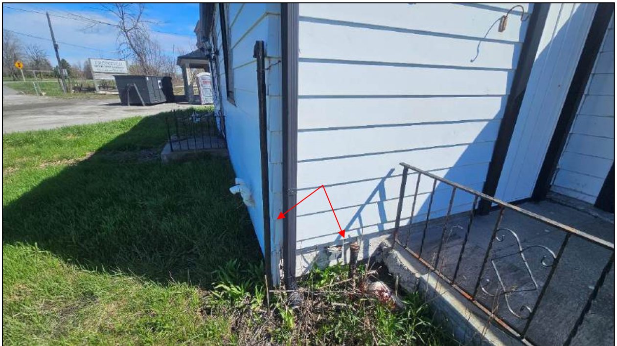
Photograph 14: View of fill/vent pipes at old building in 12371 Highway 8.
