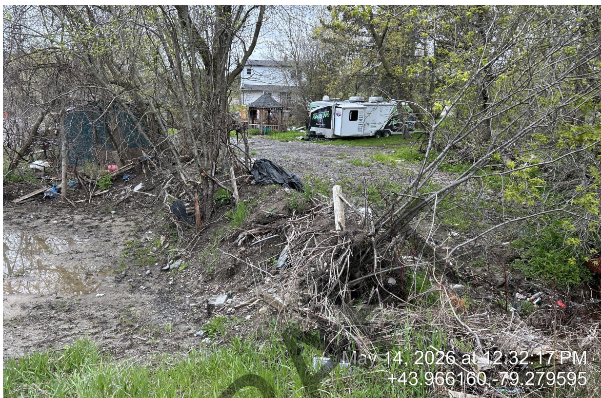
Photo 1 View of swale along the western property boundary, blocked by refuse, and surface water ponding
