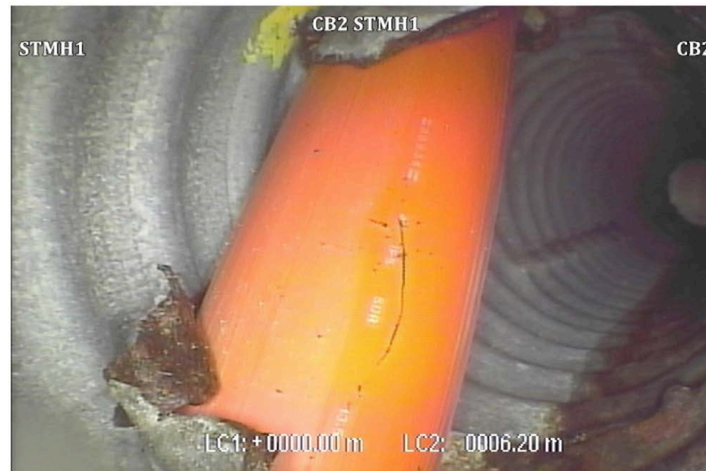
Storm Sewer Pipe Intrusion, Cross Bore
