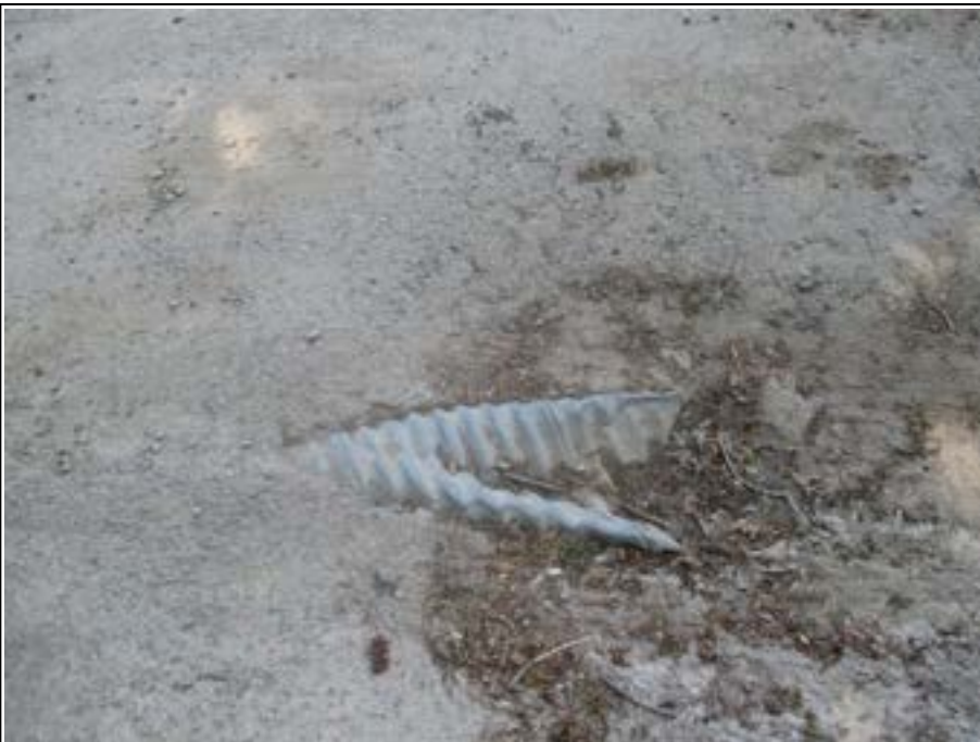
Collapsed CSP, W side Edward St. – May 30, 2018
