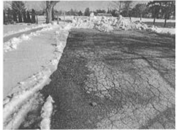
Photo 2: Edward Street looking north, showing deteriorated alligator cracking and thin asphalt layer
