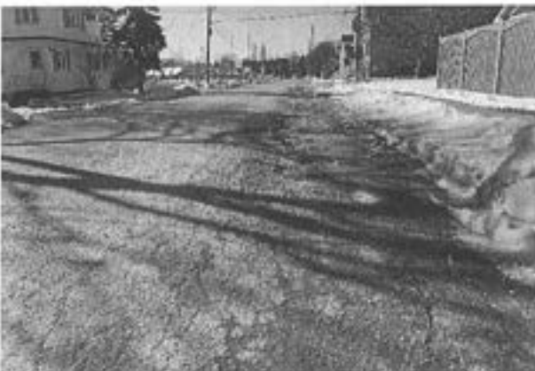
Photo 3: Edward Street looking south, showing moderate to severe alligator cracking, severe distortions and water ponding along the edge of the road
