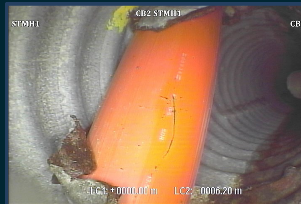
Storm Sewer Pipe Intrusion, Cross Bore
