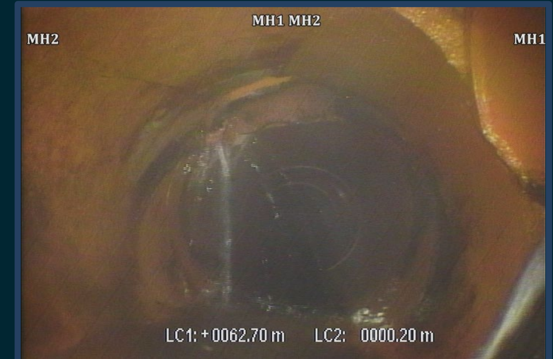
Water Infiltration Near a Maintenance Hole Connection, In Sanitary Sewer
