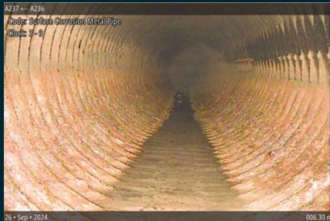
Surface Corrosion, CMP
